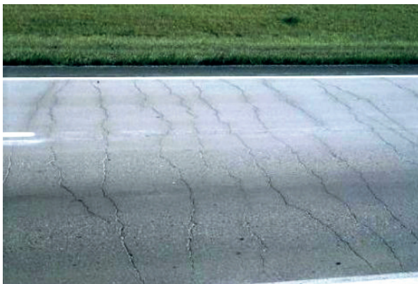
Fig. 1 Cracks that occurred in the ACP at an early age
