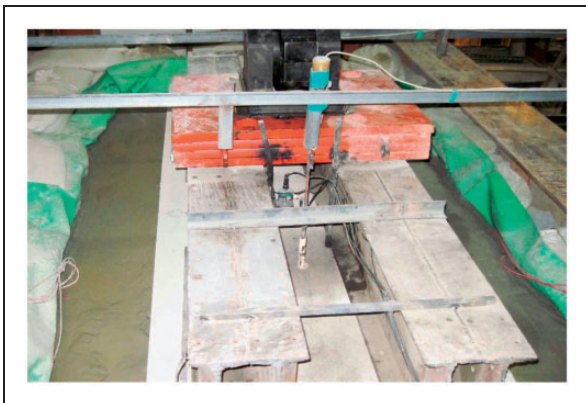
Figure 16. A large volume of slurry composed of water and fine particles squeezed out of the subgrade bed.
