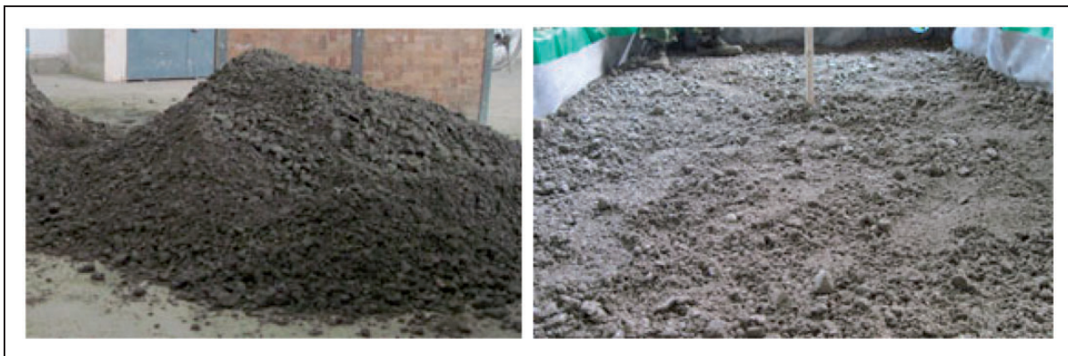
Figure 6. The graded crush stone in the optimum water content used to fill the upper layer of subgrade bed.
