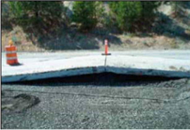
Figure 2: Concrete slab splitting off in the US [10]
